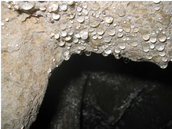
Figure 2. Condensation in CSB passage.
